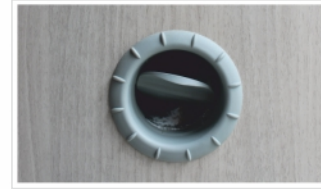
Heating outlet duct
