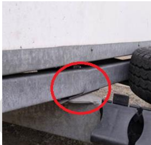
Photo 2. Broken beam that has been damaged due to overloading - defect cannot be claimed
