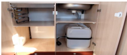
Photo 36. Water tank (to the right and valves to the left)
