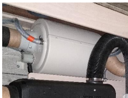
Photo 24. Water heater, 5l.
